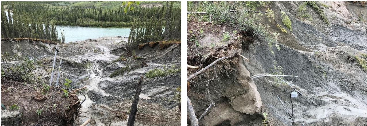
Figure 7. WH_1456_BH3 (BH3) failure, image taken on August 13th 2020
