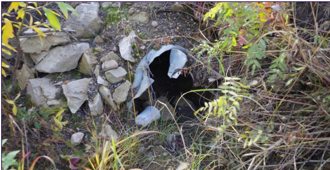
FIGURE 6.2.1. EXAMPLE OF A CULVERT THAT IS DAMAGED AND UNLIKELY TO SERVE AS DESIGNED.
